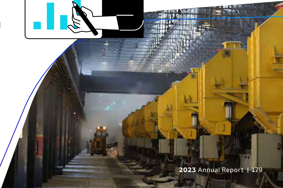
Pot Room 3, Alumínio (SP) plant
